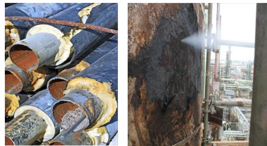
Detrimental effects on CUI. Courtesy: https://www.eddyfi.com/oil-gas/corrosion-under-insulation-plague-what-you-need-to-know/
