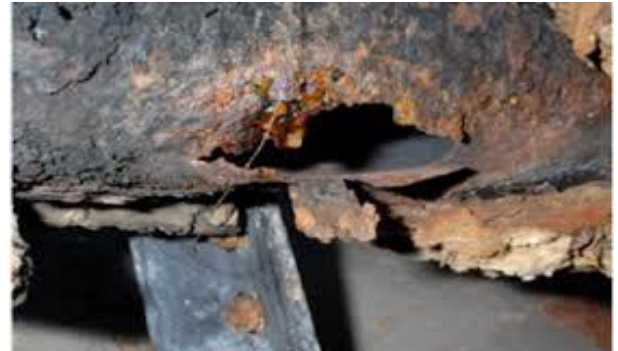
Corrosion under insulation found on pipe. Courtesy: https://www.alsglobal.com/myals/news/2017/06/asset-care-counts---corrosion-under-insulation
